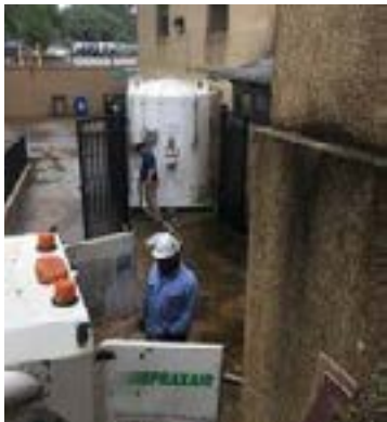
Left F4: Praxair's Marvin does the first fill of the exterior supply tank from the cryoshuttle.
