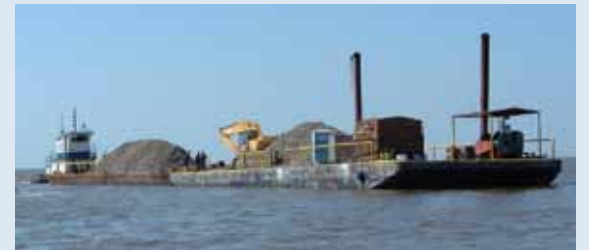
Creation of an artificial reef typically involves barges that transport the reef material to the construction site.
