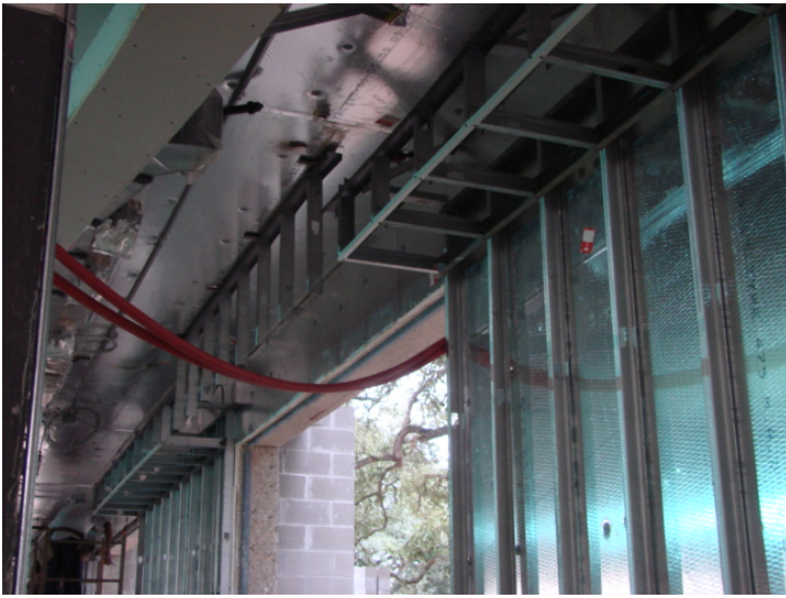
9. Metal fur down work continue along the south wall of the lounge.
